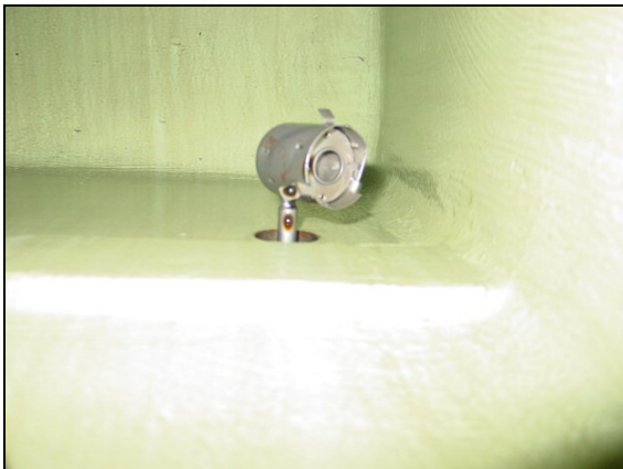
Fig. 3: A twisted suction funnel, as shown here, lets through excessive oil and can cause false alarms and clogging of OMD
